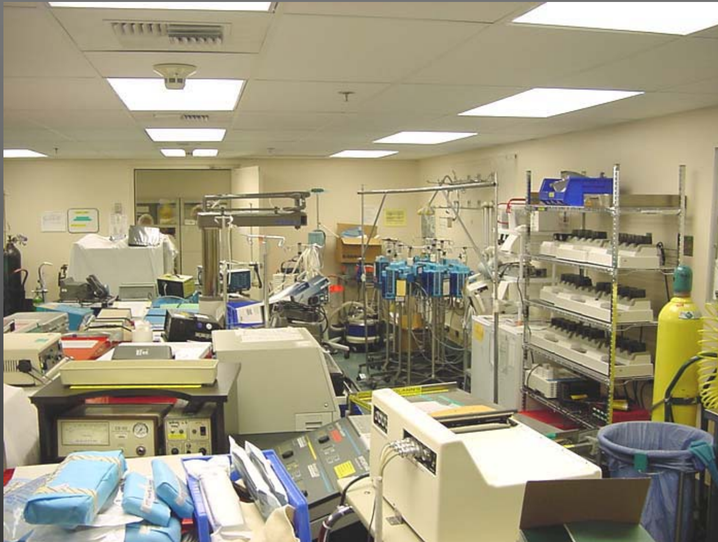
OR Equipment Room Before 5S
